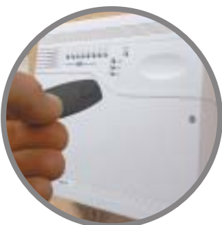
Setting the System
