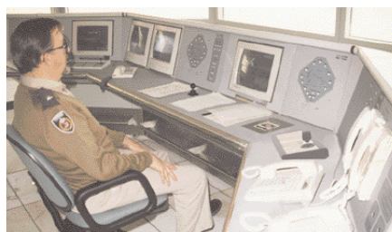
Control Console Layout with General MIMIC Panel, Alarm MIMIC & Radio Link
