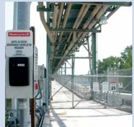
By identifying and controlling who enters and exits the facility, the site is better protected.
